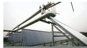
By using the solar power collecting device installed on the roof of the rest area, warm water is supplied to customers 24/7 without causing environmental pollution
